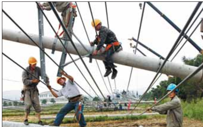
Electricians repair fallen lines after the typhoon blew down electricity poles in Wenling, Zhejiang province, on Wednesday.
