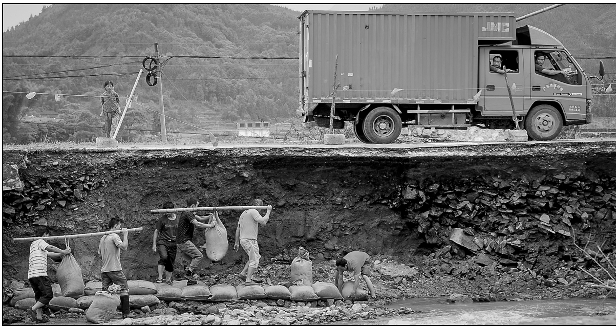
Residents repair a road damaged by flooding in Sanfang, a township in Liuzhou, Guangxi Zhuang autonomous region, on Saturday after the region was hit by heavy rain. PROVIDED TO CHINA DAILY
