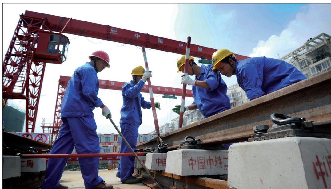
Workers install the metro rails in Chengdu. The capital is expanding its metro line network linking satellite towns with its central area.
